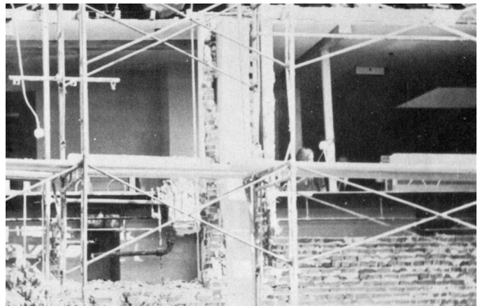
Figure 25c Damage to exterior wall of a laboratory at LACC’s Glendale campus, 1971.
